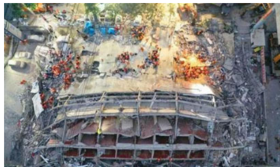
Figure 2. Xinjia Hotel steel structure collapse
